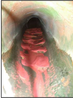
Fig. 11 Coarse sediment deposited in outfall pipe
